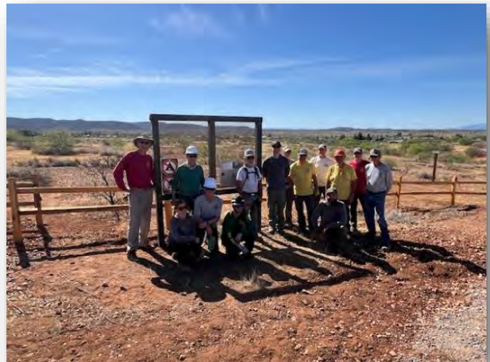
Kiosk installation at the new E. Willow Pt. Rd. trailhead in Cornville
